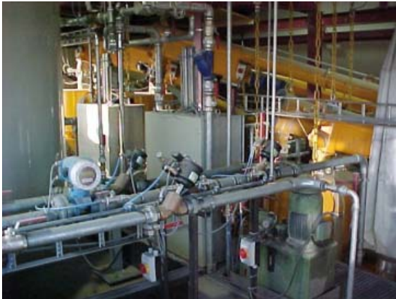
Figure 4: Hot and cool water installation
