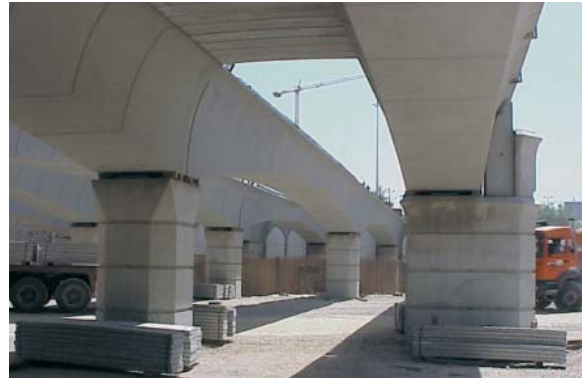
Fig. 30: Stock of non recoverable slabs
