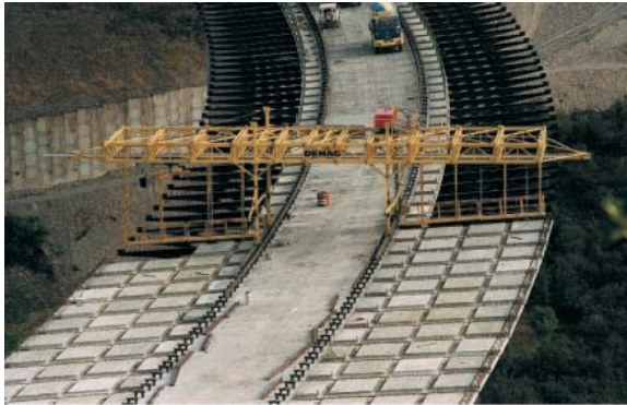
Fig. 34: Precast deck slabs of full thickness on steel structure (box girder & diagonals)
