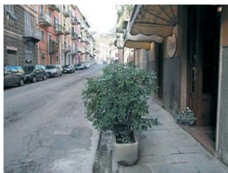
Figure 2: typical deteriorated pavement on a urban local road.
